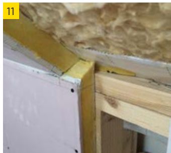
10 Ensure that adjoining boards are flush with each other before beginning to fix the boards to the studs. Use a continuous line of screws across both top and bottom boards.
