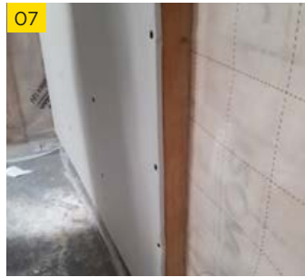
07 Ensure that the dry lining screws on the joints are inserted into the stud as straight on as possible to enable a flush finish and are screwed into place within 13mm of the InLiner Spacer Screws.
