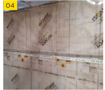
04 Seal any seams between the Vario Membrane with Vario KBI Tape. Any tears in the membrane envelope should also be sealed with Vario KBI Tape, to ensure an airtight envelope is maintained.
