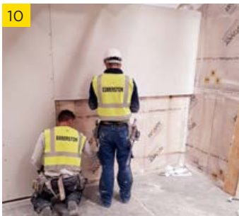
09 Boards can be installed horizontally or vertically. If installing horizontally, ensure that the top of the board is lined up with the perimeter stud at the top of the knee wall.
